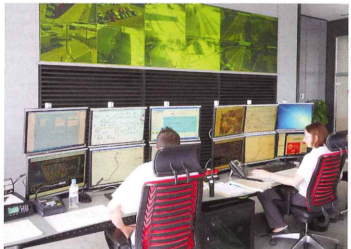
▲ Two duty controllers monitor the entire length of Line 1.
